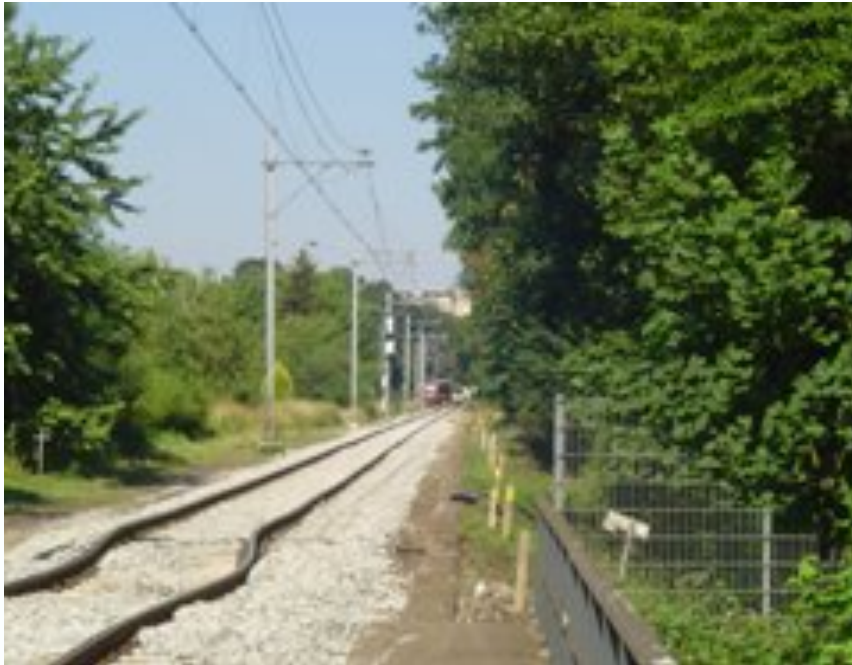
THERMAL BUCKLING OF RAIL TRACKS DUE TO HEATING BY SUN (SUN KINK)
