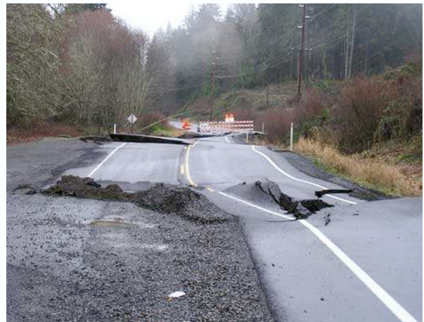
ROAD BUCKLING DUE TO TECTONIC COMPRESSION OF SUBSTRATE
